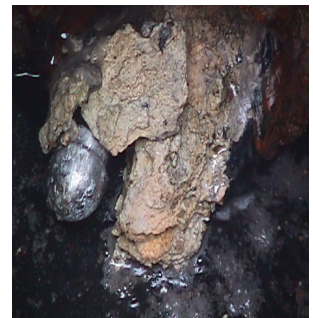
A picture is worth a 1000 words. Solid chunks of grease & soap in a local school's main line. The entire line was almost closed off. The students did not like that we were able to clean the line and keep the school open.
